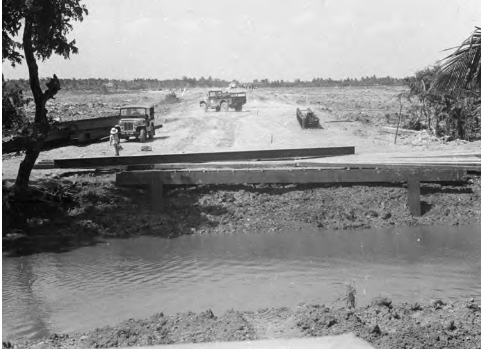
Despite delays caused by Operation SPEEDY EXPRESS, the 34th Engineer Group continued to make progress along Highway 4.
